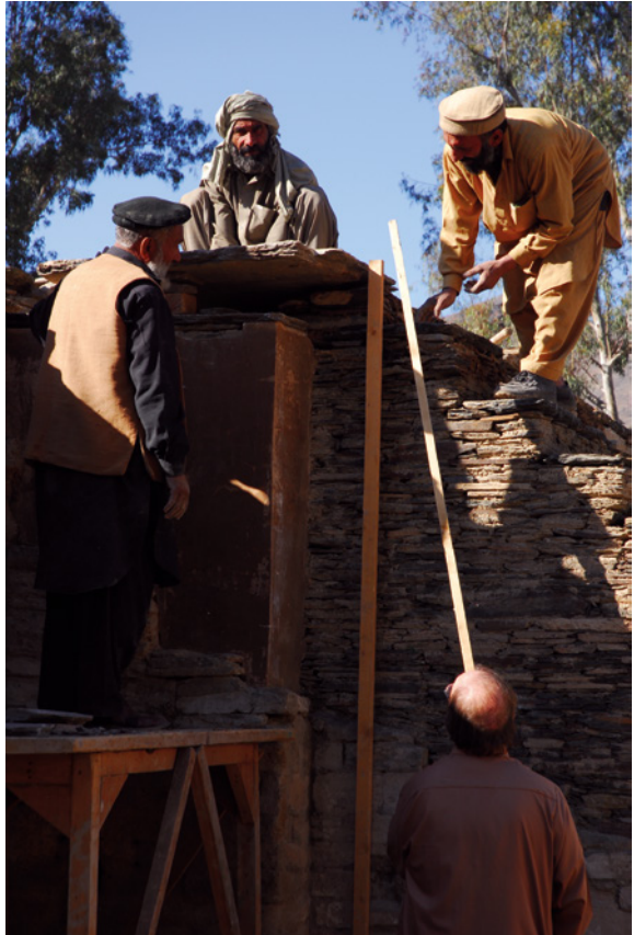
Figures 2-3 Restoration in progress at Saidu Sharif I. 2012 (ACT; photo by Fabio Colombo)
