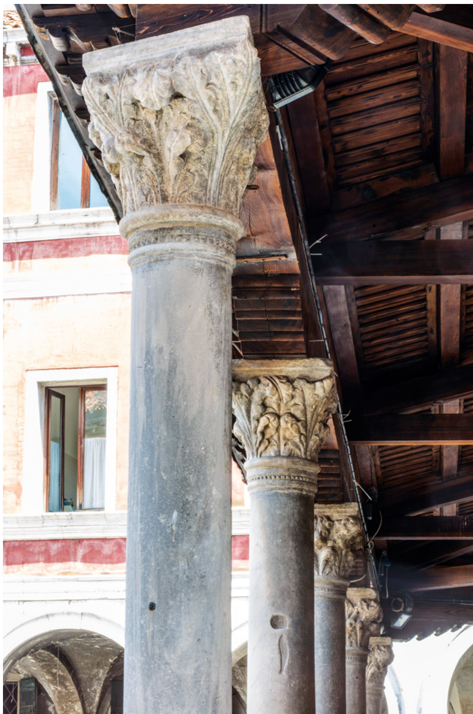
Figure 16 Venice, Rialto, Church of San Giacomo. Lateral view of the portico. Detail. Photo © Böhm
