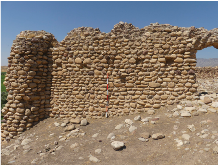
Figure 9 Regular banks of the masonry (eastern external wall)
